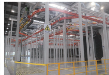
● 智能输送 Installation conveyor
