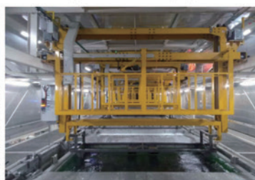
● 车架电泳线 Automotive chassis E-coating line
