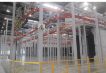
● 智能输送 Installation conveyor
