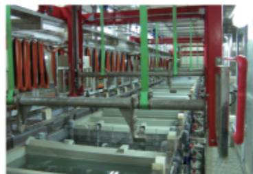
● 氧化/磷化设备 Oxygenation equipment Phosphorization equipment
