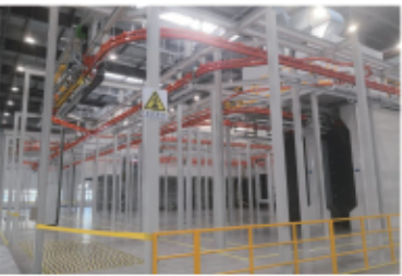
● 智能输送 Installation conveyor
